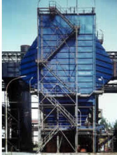
Figure 2.1: Precipitator used to Control Emissions from a Wood Fired Boiler
