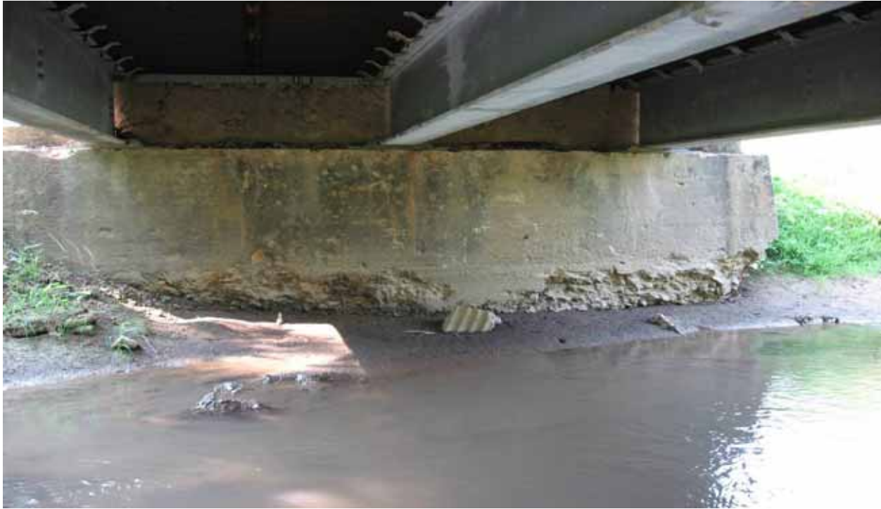
Figure 3.19: Disintegration of Concrete on the north abutment
