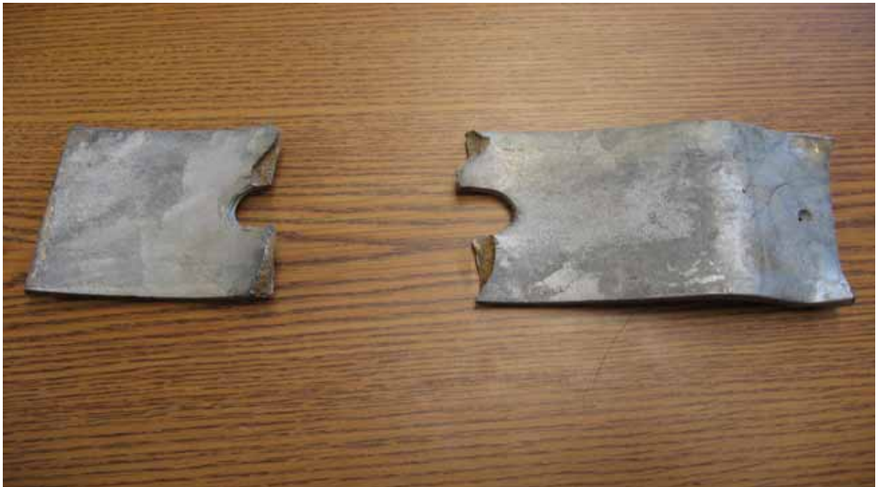
Figure 3.17: Failure Mode of a Stringer to Deck Connector on Hackers Creek Bridge
