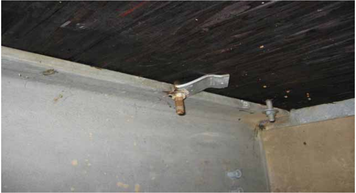
Figure 3.16: A Failed Stringer to Deck Connector on Hackers Creek Bridge
