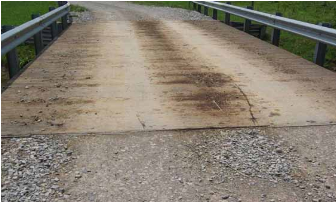
Figure 3.6: Wheel Path Rutting of the Deck on Peel Tree Bridge
