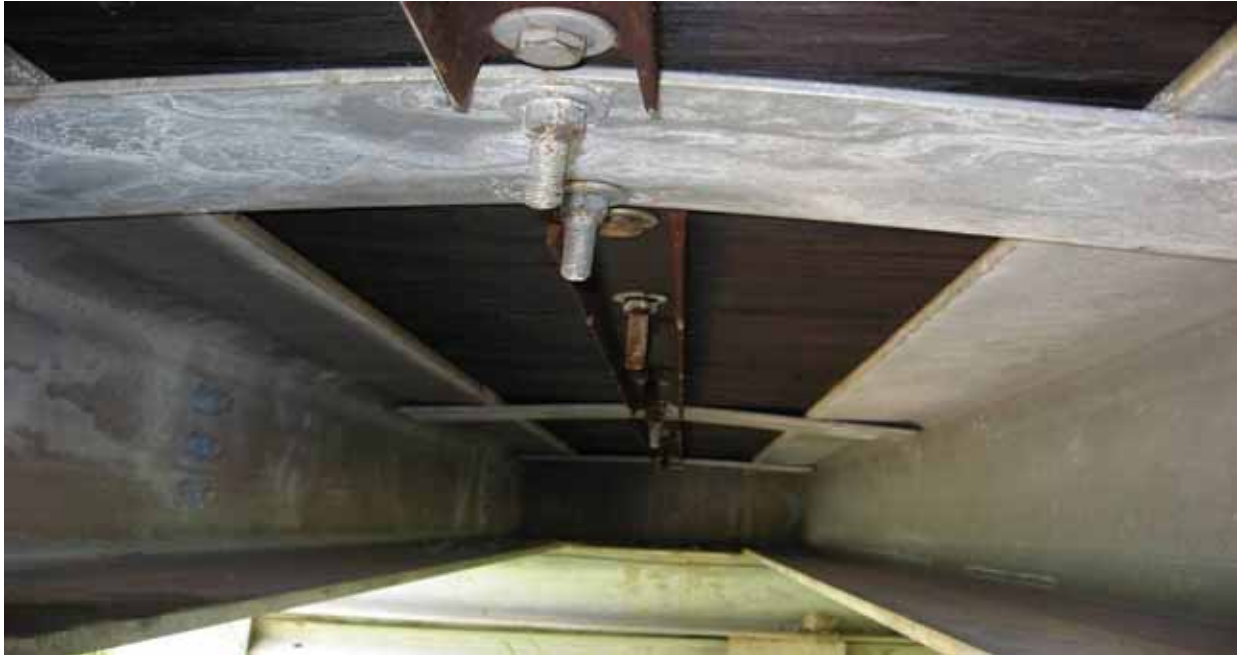
Figure 3.11: Conditions at the Bottom of Peel Tree Bridge
