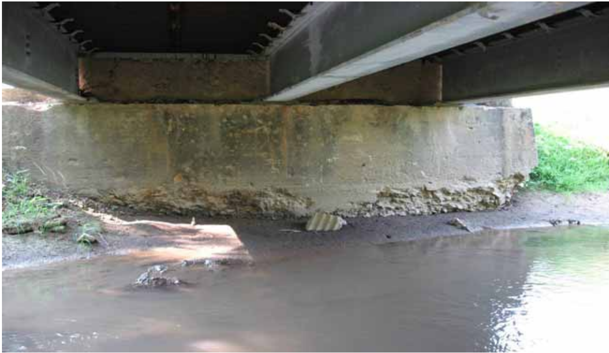
Figure 3.19: Disintegration of Concrete on the north abutment
