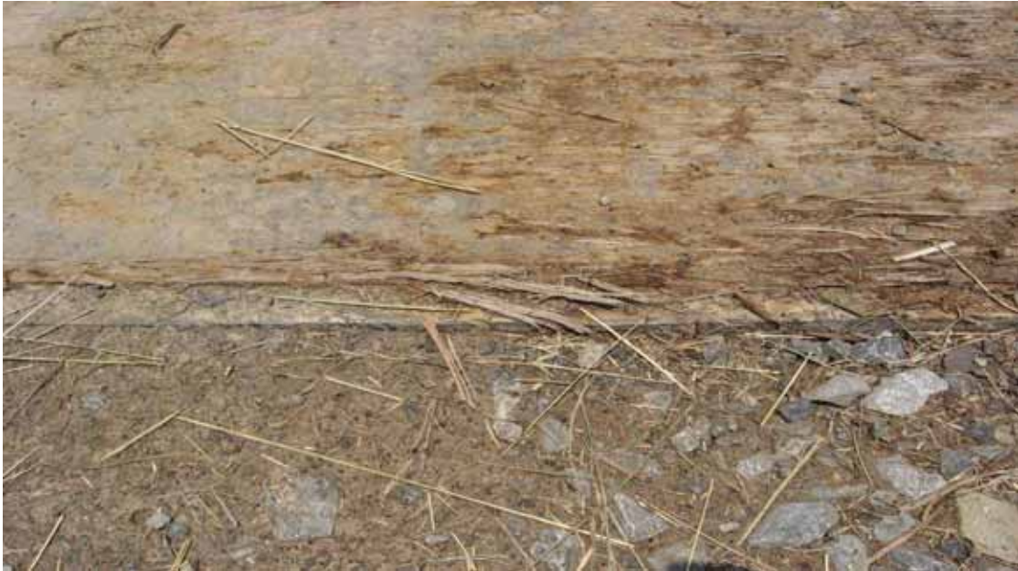
Figure 3.7: Parallam Deck Chipping on Peel Tree Bridge
