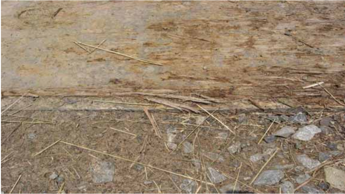
Figure 3.7: Parallam Deck Chipping on Peel Tree Bridge
